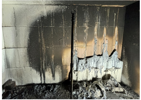
POST-TEST (RIGHT SIDE WALL)
